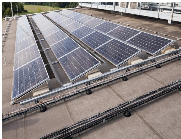
Figure 10 Example of rooftop solar installation
